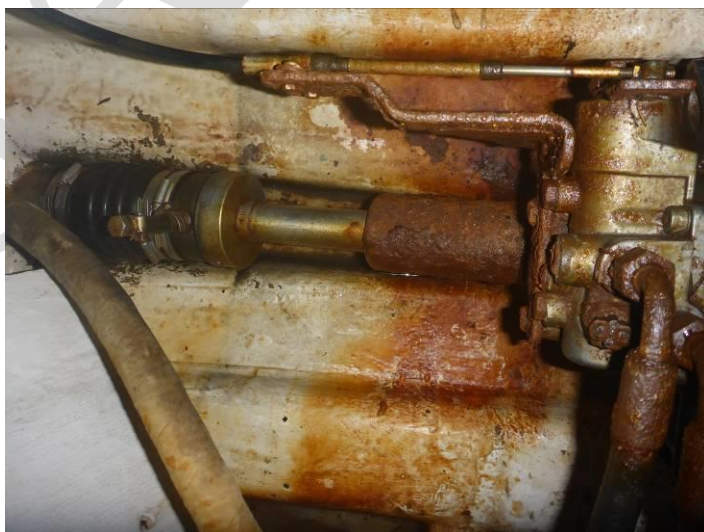
Engine rooms would benefit from some cleaning and couplings require treatment / paint
