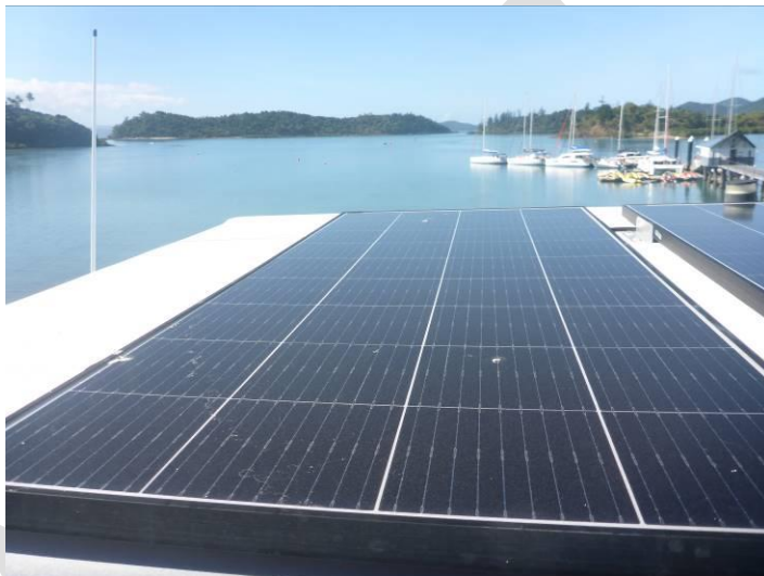
New solar installation will assist battery management
